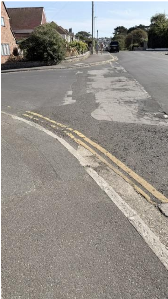
No drop curbs at this junction
