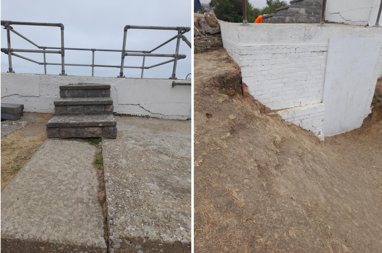
Figure 2:a) Subsidence behind the tunnel. b) Staff room showing depth of rooms below ground level.
