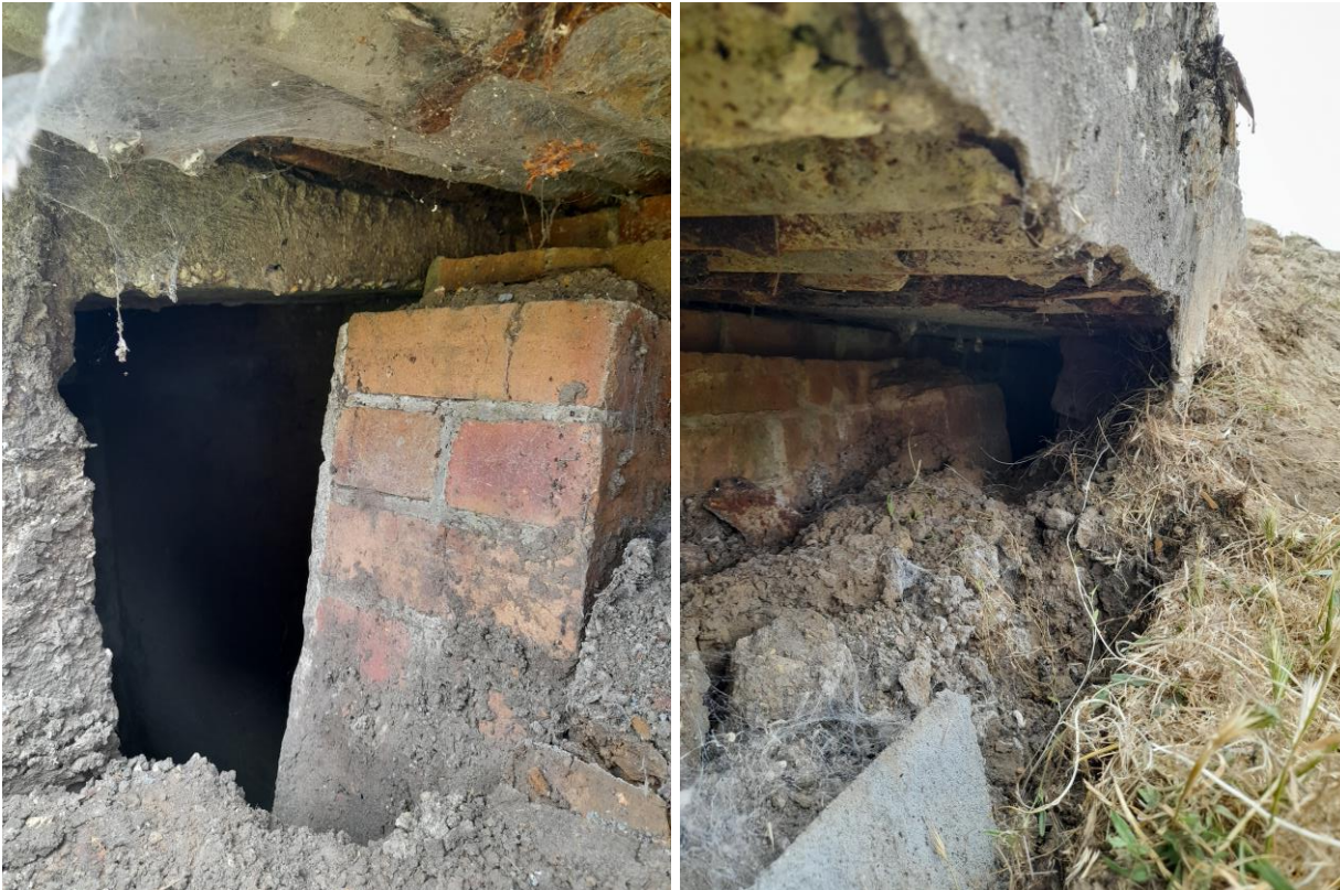
Figure 1:a) Voiding created by damaged wall. Looking into front room. b) Displaced northern wall, showing it leaning on the southern wall
