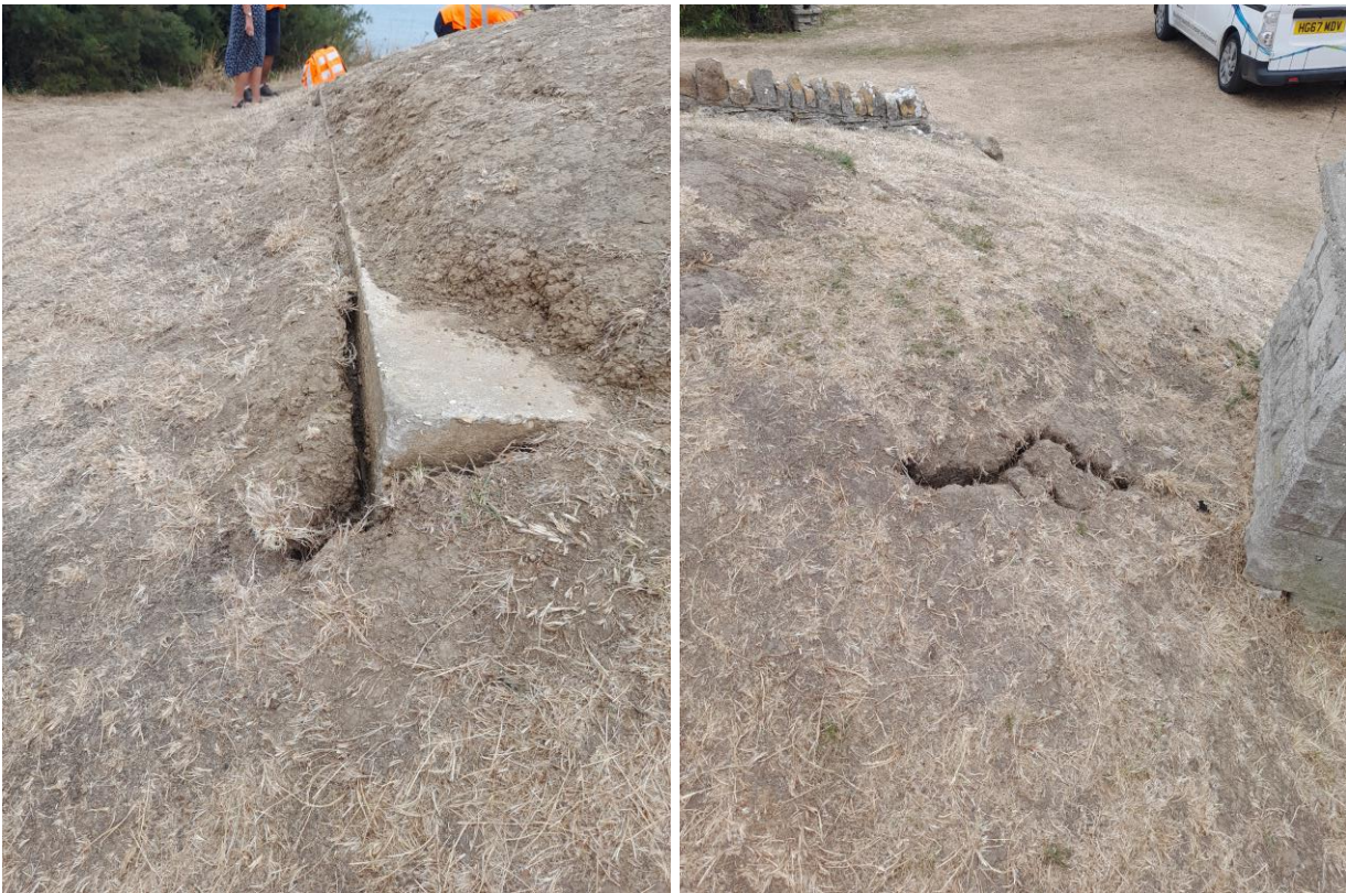
Figure 3: Desiccation and tension cracking in earth placed on top of ammo room
