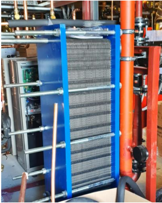
Plate heat exchanger
