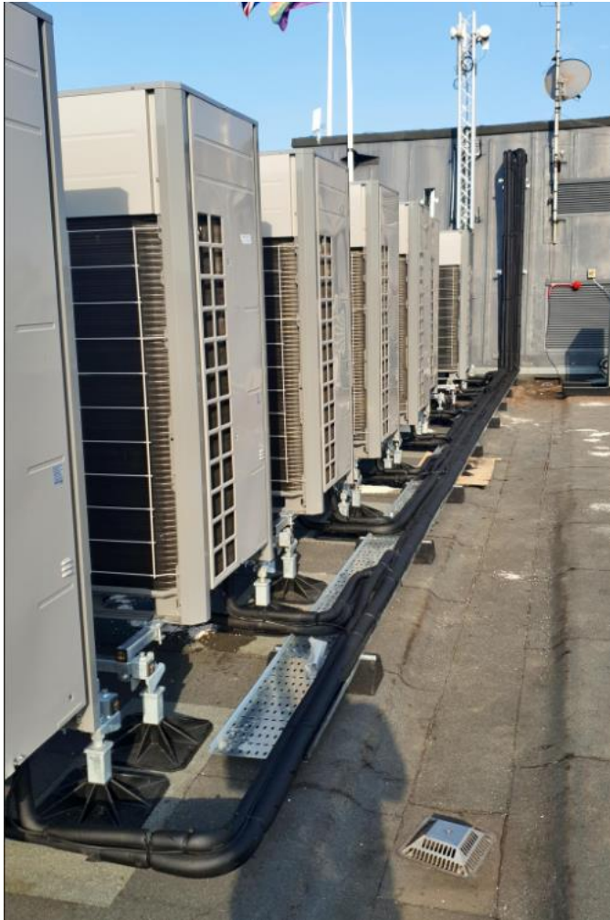
External Therma V units
