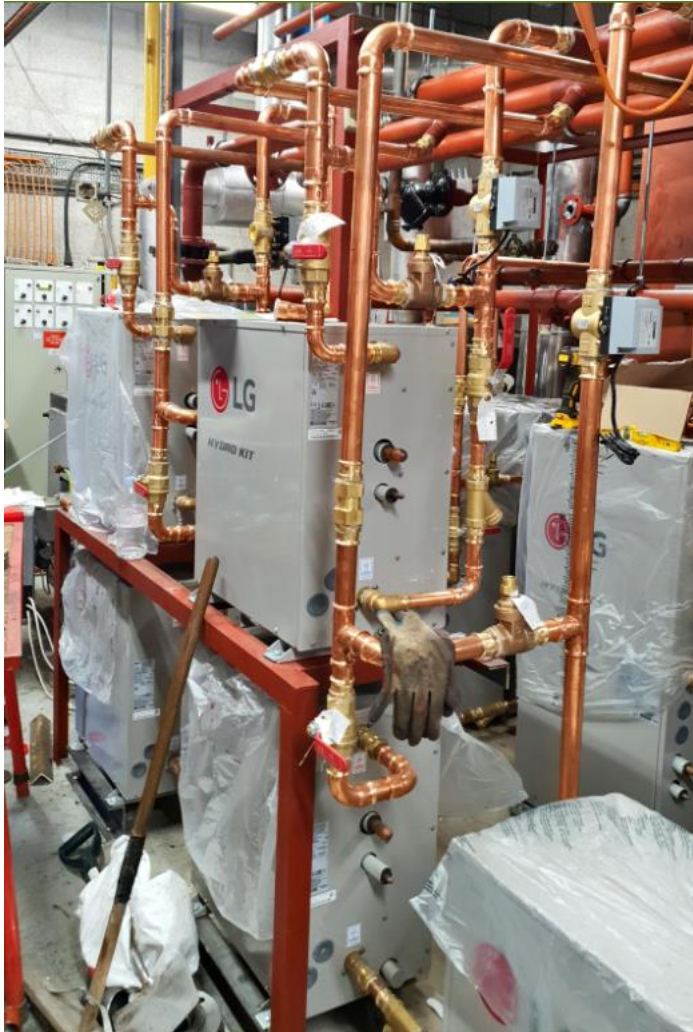
Hydro boxes – transferring heat from outside
